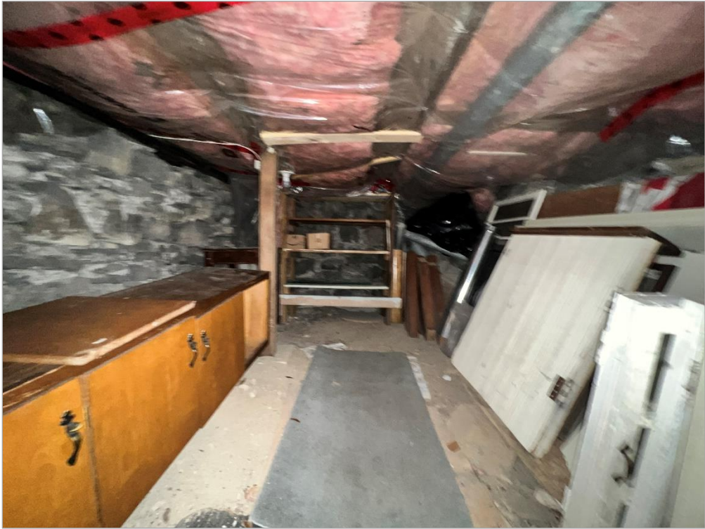
Storage and mechanical room
