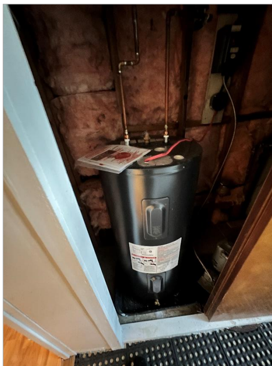
Hot water tank
