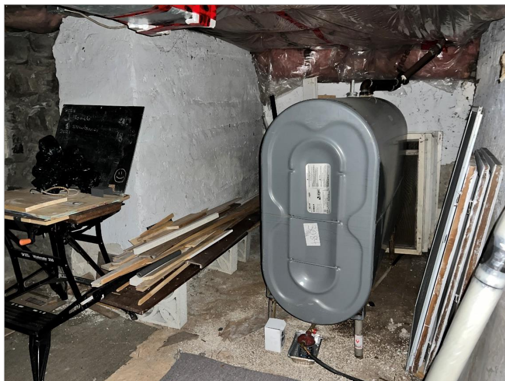
Storage and mechanical room
